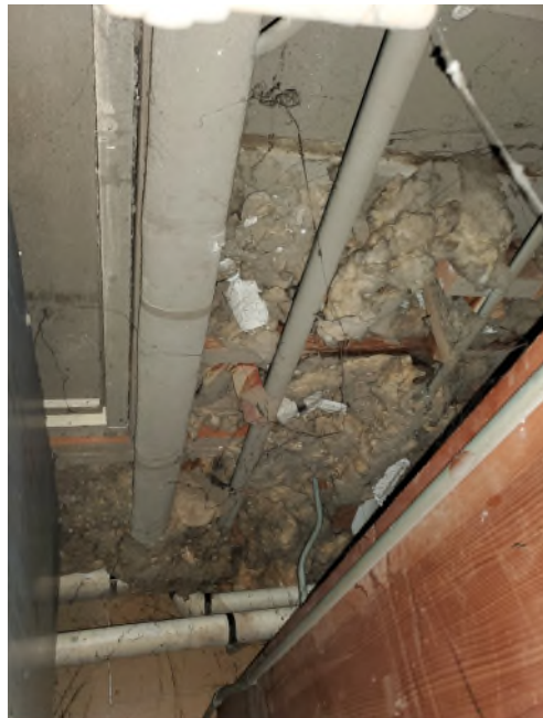
View of 4" Thermal System Insulation (TSI) Pipe Run
