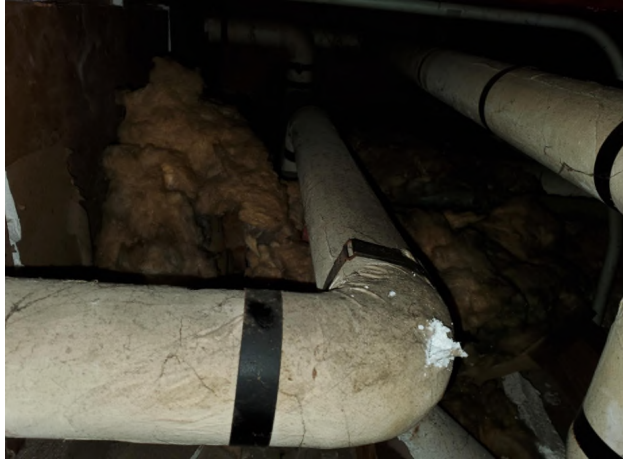
View of 4" Thermal System Insulation (TSI) Elbow
