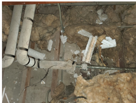
View of Debris
