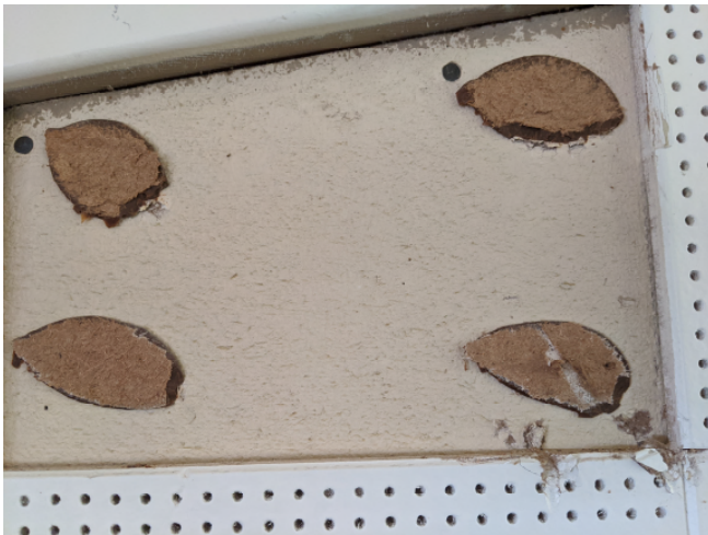
View of 1'x1' Ceiling Tile with Hockey Puck Mastic
